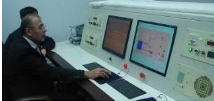
Fig. 2. The control room of the subcritical reactor laboratory at the nuclear engineering department in Jordan
