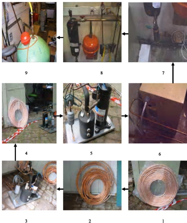
Fig. 4. Showing preparation of coils (1-2), installation of heat pump (3-6) and connection of water supply system (water pump, flow metre, expansion valve and the boiler) (7-9)
