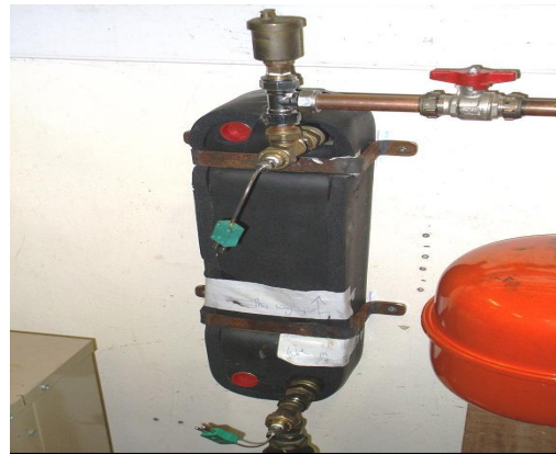
Fig. 14. Shows the heat exchanger
