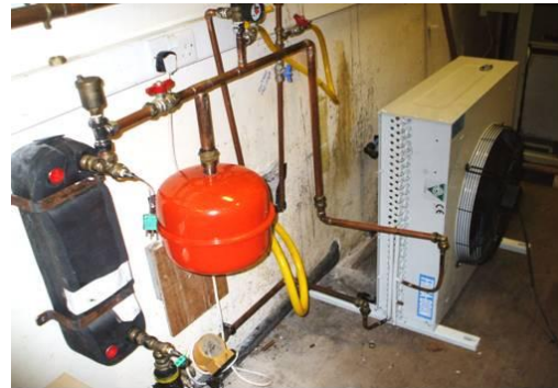
Fig. 15. Shows the connections of the heat exchanger, water pump, heat rejection fan and expansion valve
